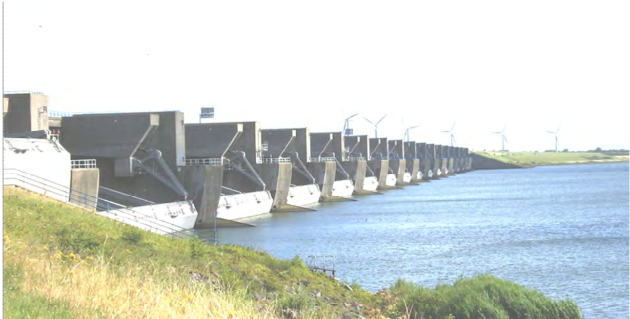
Plate 2: The portion of the Haringvliet Dam indicating where the Rhine River empties into the North Sea (the Rhine River lies to the right side; the shot was taken by the Author during a study trip in 2008).
