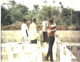
Construction of snail pen at the rural development centre, in Imo State
