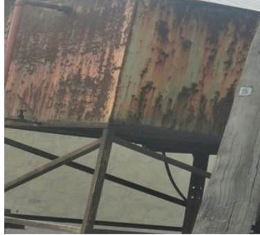
corroding storage tank
