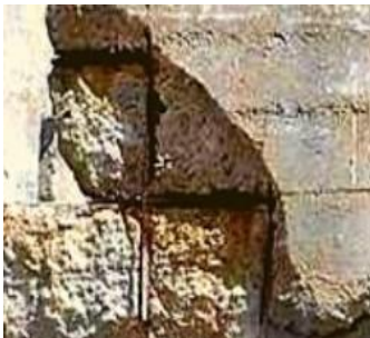
Corrode rod in a building
