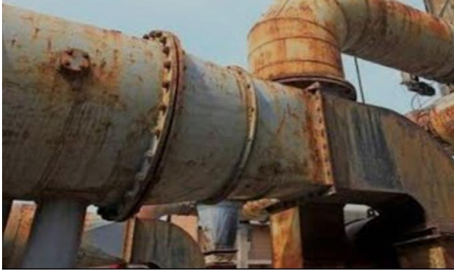
Plate 4. A corroding Oil and Gas installation. Photo: credit appmfg.com
