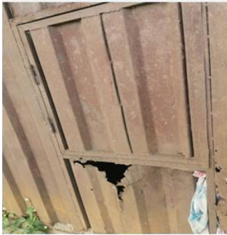
Corroded metal door
