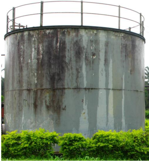
Figure10b Vertical 100 ton palm oil storage tank
