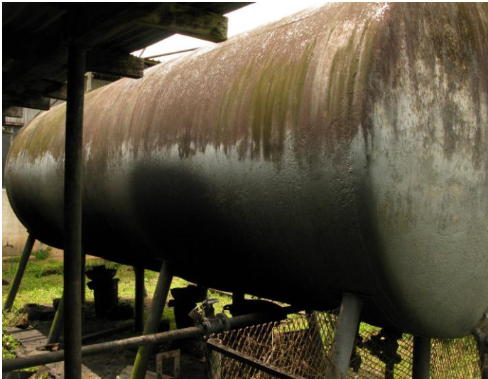
Figure 10a Horizontal 20 ton palm oil storage tank
